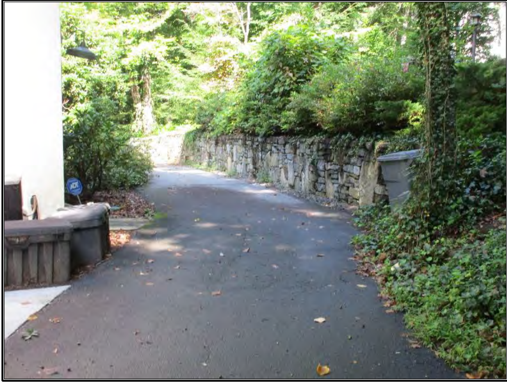
Figure 223. View of driveway encircling the house to the north along the rear retaining wall.
