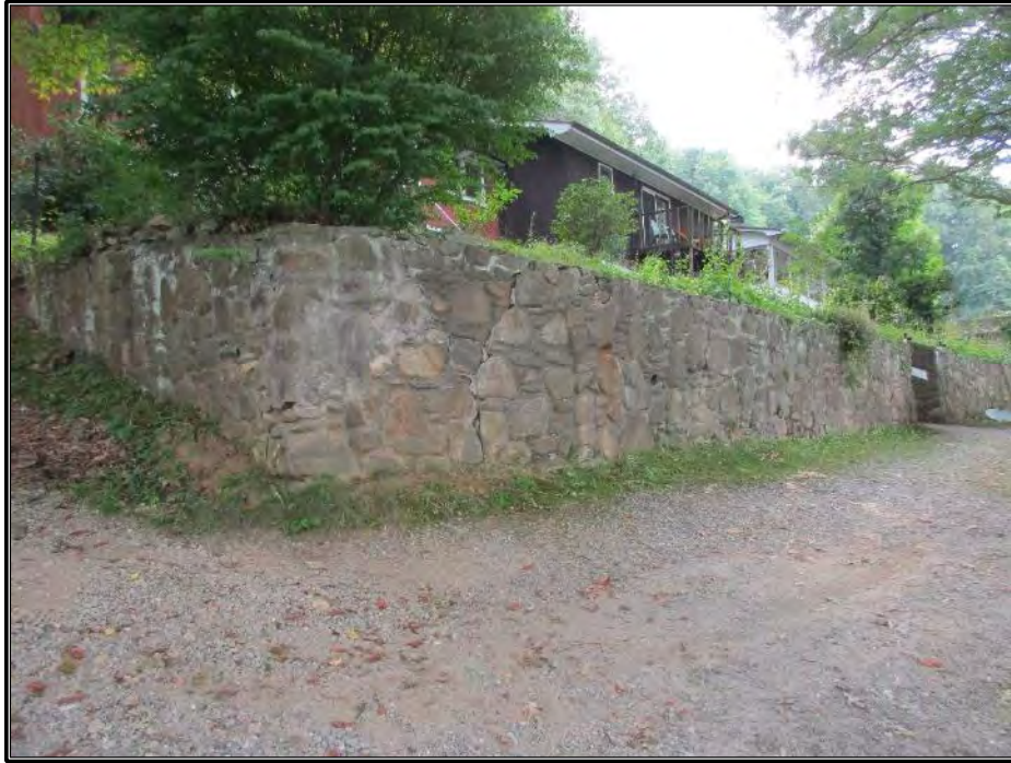
Figure 187. Stone retaining wall along service road and gravel drive with stair entry.
