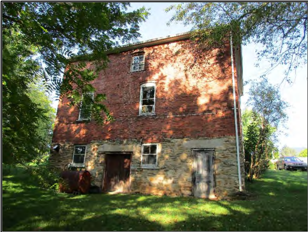
Figure 398. Rear (eastern) elevation of the carriage house with entry to the stables.
