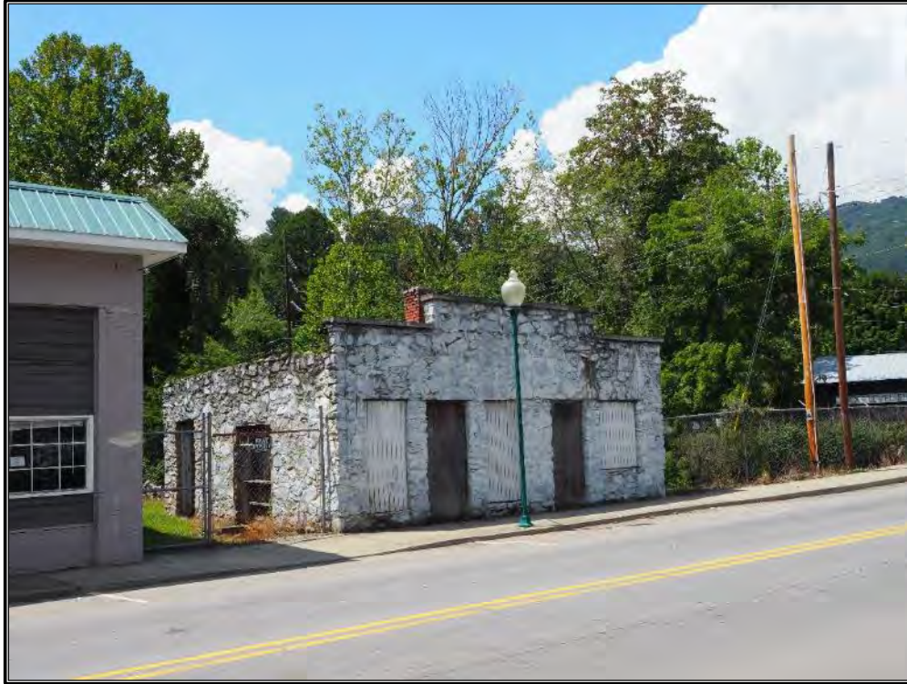
Figure 73. Rubble-rock masonry, circa 1940 commercial building in Frog Level, just west of the Waynesville Main Street Historic District (HW0161) on Depot Street adjacent to Richland Creek.
