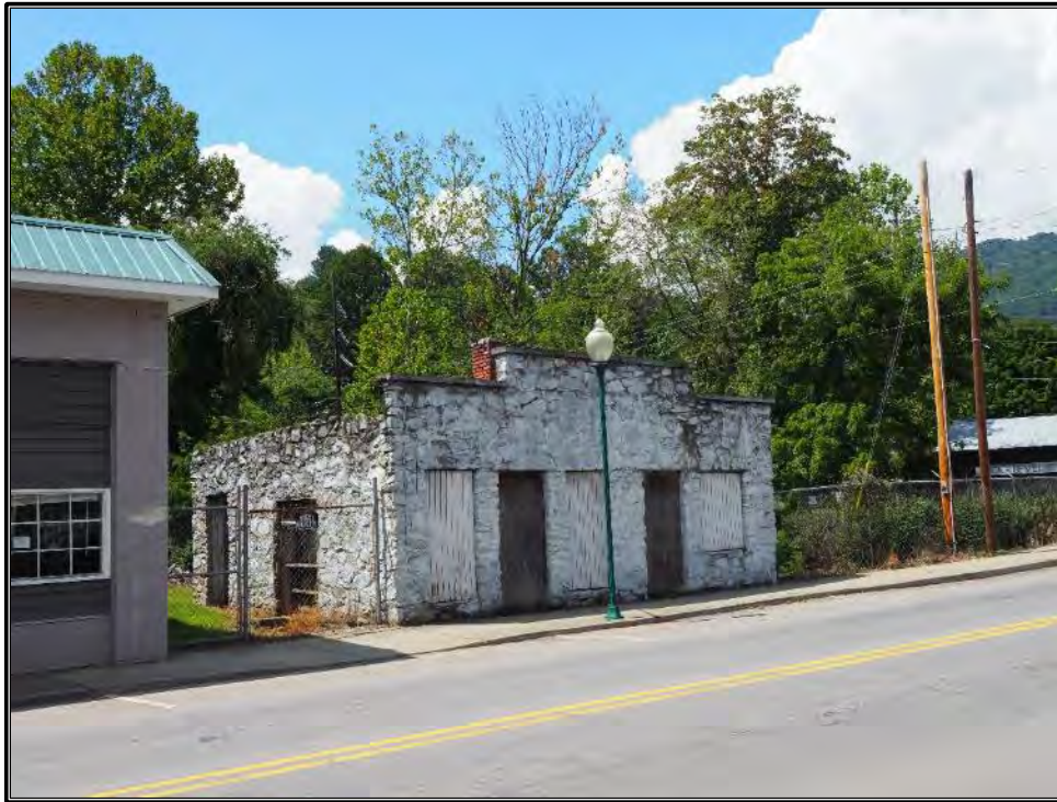
Figure 42. Rubble-rock masonry, circa 1940 commercial building in Frog Level, just west of the Waynesville Main Street Historic District (HW0161) on Depot Street adjacent to Richland Creek.
